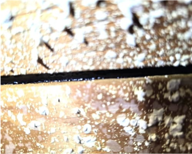
Photo 1 - Secondary Water Resistance
