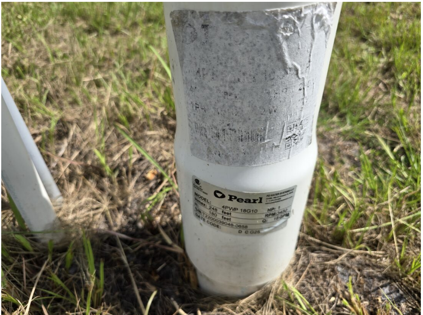
Placa de bomba de pozo Pearl / Pearl well pump data plate
