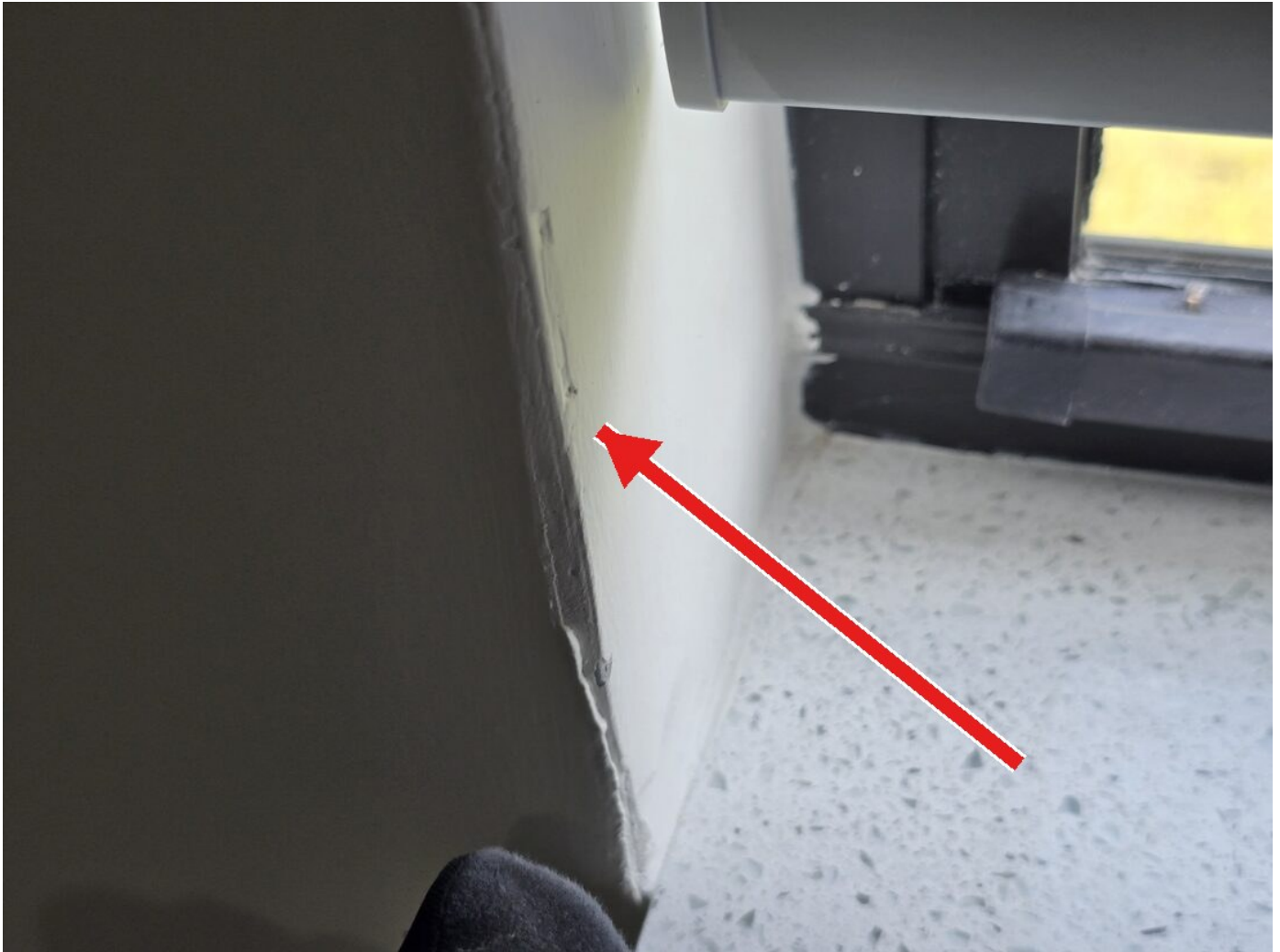
Esquina sin acabado completo / Corner with incomplete finish
