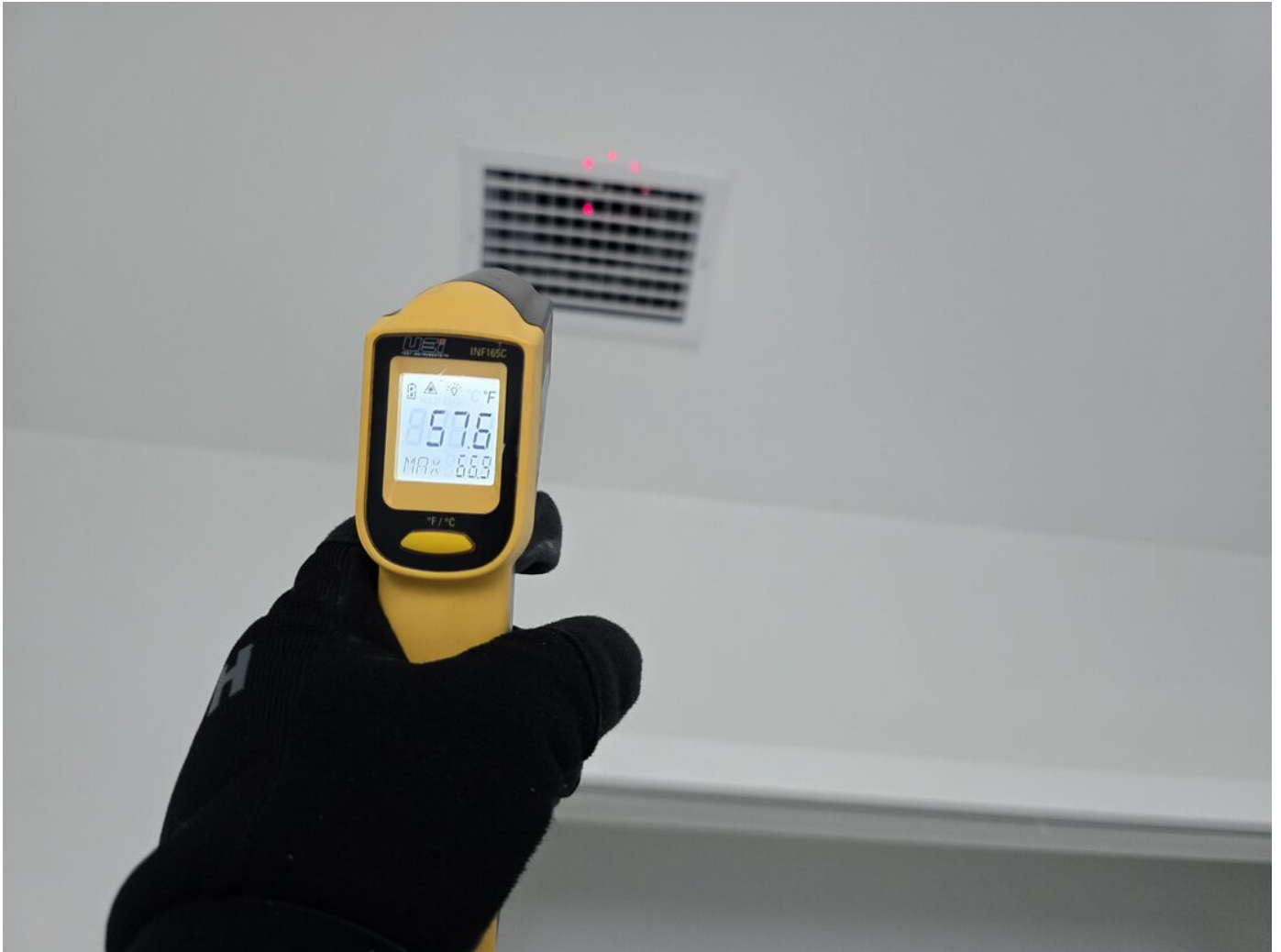
Lectura infrarroja en difusor / Infrared reading at diffuser
